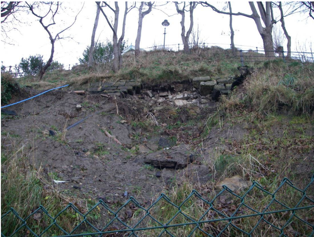
Plate 30 Site view of retaining wall and slope failure behind The Spa on Spa Cliff.
