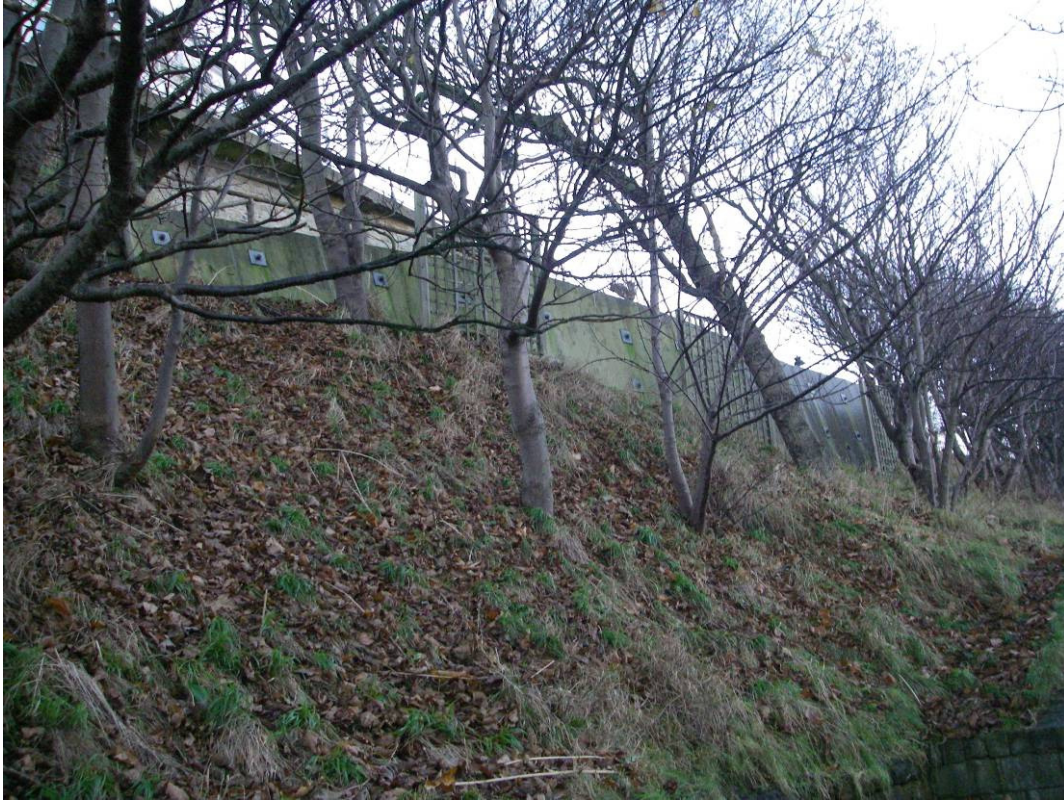
Plate 27 Site view of slope crest retaining walls at Prince of Wales Cliff.
