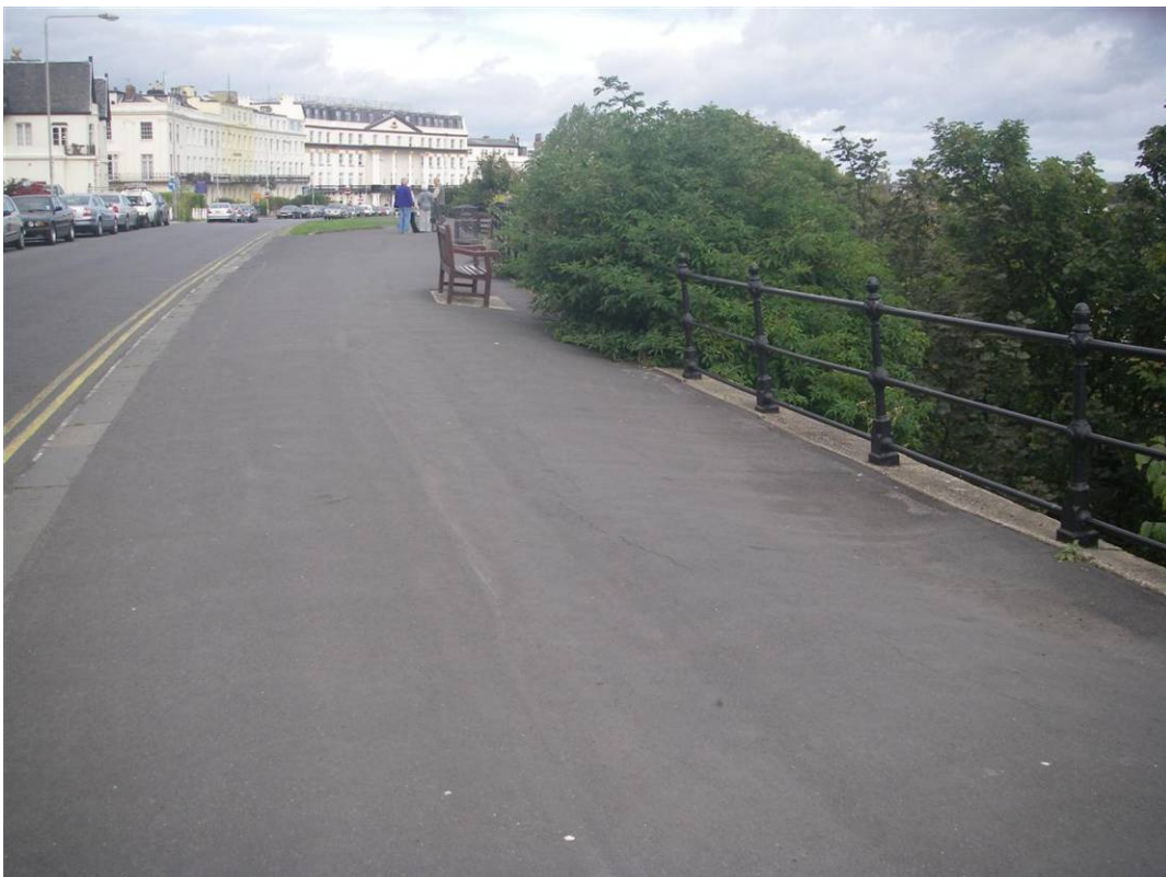
Plate 68 Scarborough South Cliff Promenade showing signs of subsidence.
