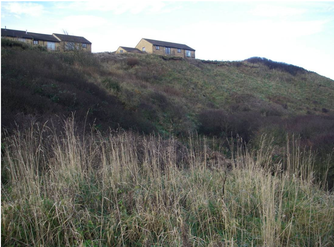
Plate 12 Site view of Behaviour Unit II showing over steepened back-scarp below Upper Plateau.
