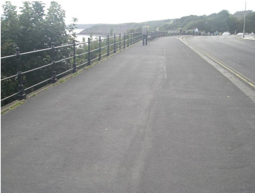
Plate 69 Scarborough South Cliff Promenade showing signs of subsidence.
